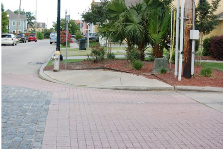
Figure 3: ADA curb ramp with dead end sidewalks
