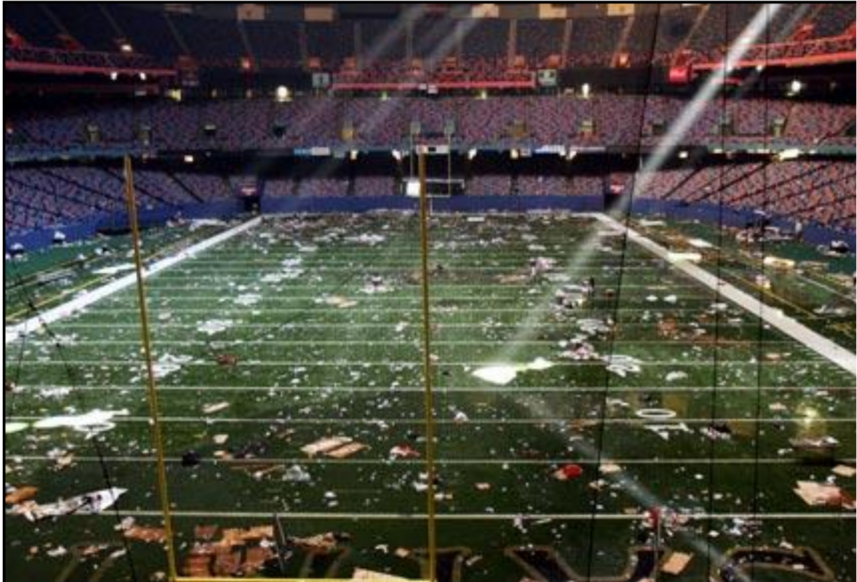
Hurricane Katrina and evacuees caused over one hundred million dollars in damages to the Superdome. (Photograph courtesy AOL News)
