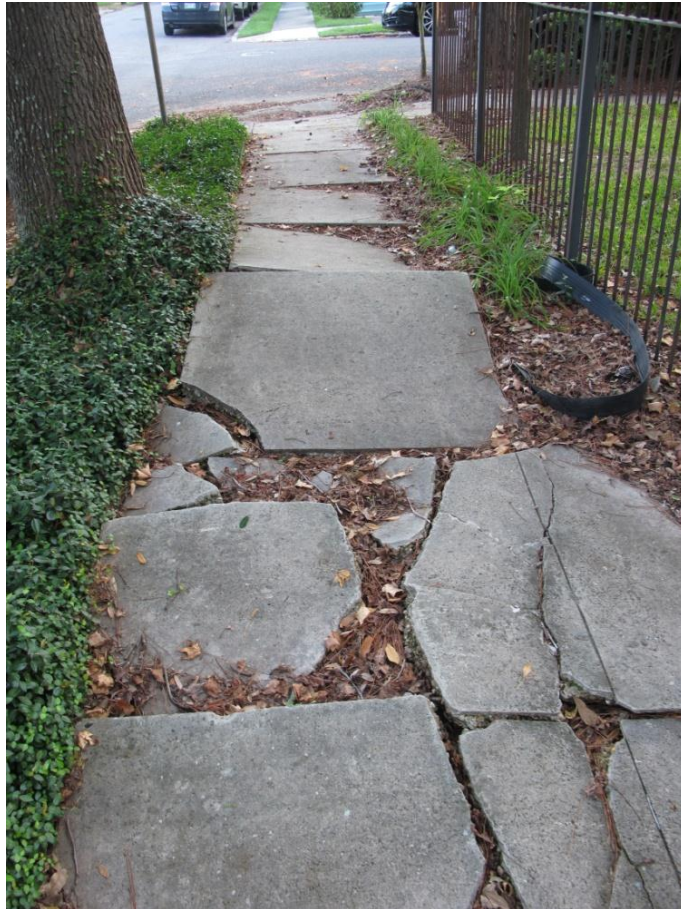
C3= Root-Damaged sidewalk in Short Street
