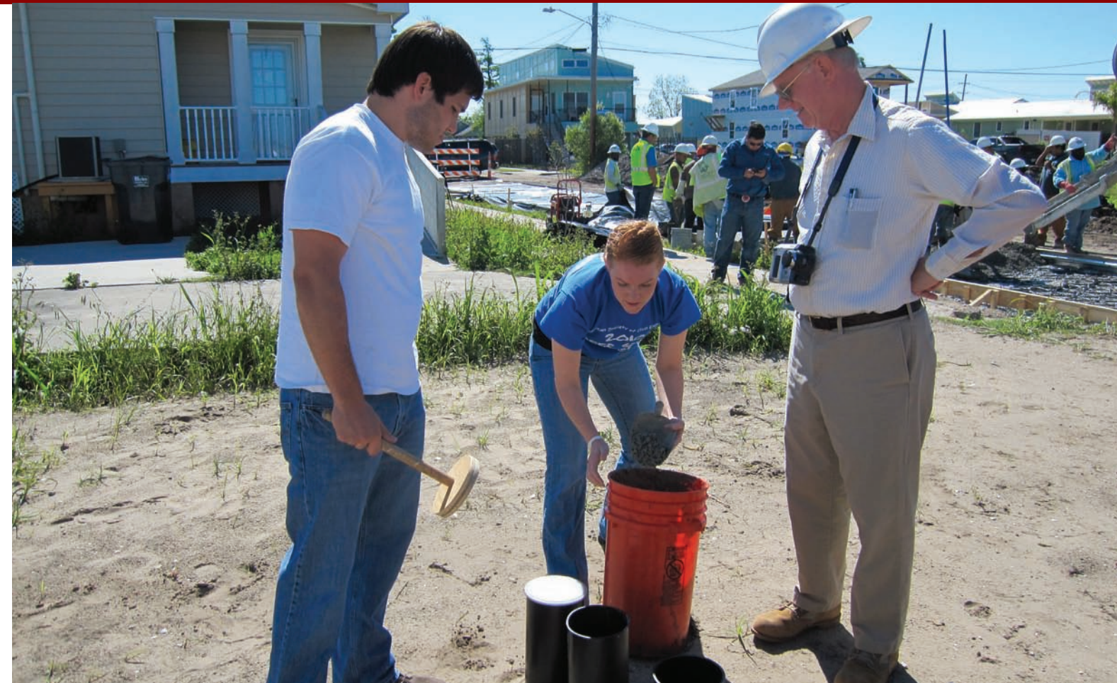
As workers pour the section of street that they designed, civil engineering students Matt Zeringue and Anne Heath take concrete samples while instructor Chuck Fromherz looks on.
