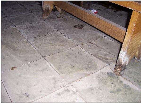
Floor tile damage, The Cove
