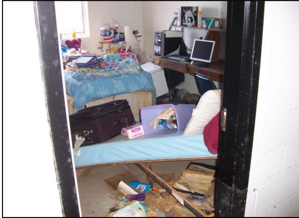
Water damage, Bienville Hall student room
