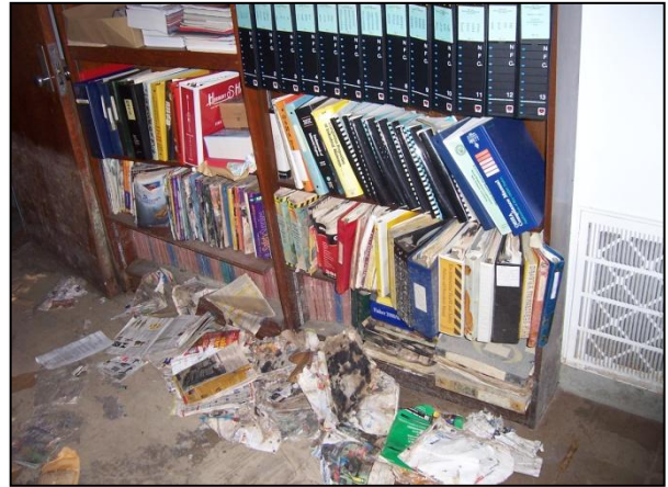
Water damage, Facilities Service office
