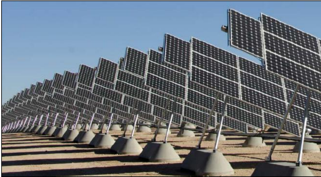
Figure 6.3: A View of Nellis Solar Power Plant, Nevada. [Source: Ref 31] (The single axle trackers can be seen attached to the solar panels)
