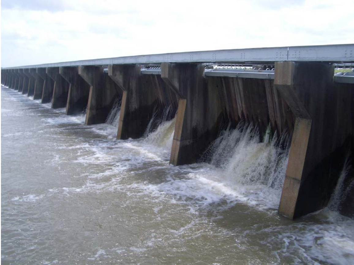
Figure 2.2 Photo showing leakage through the weir at the Bonnet Carré Spillway on April 11 th , 2008.
