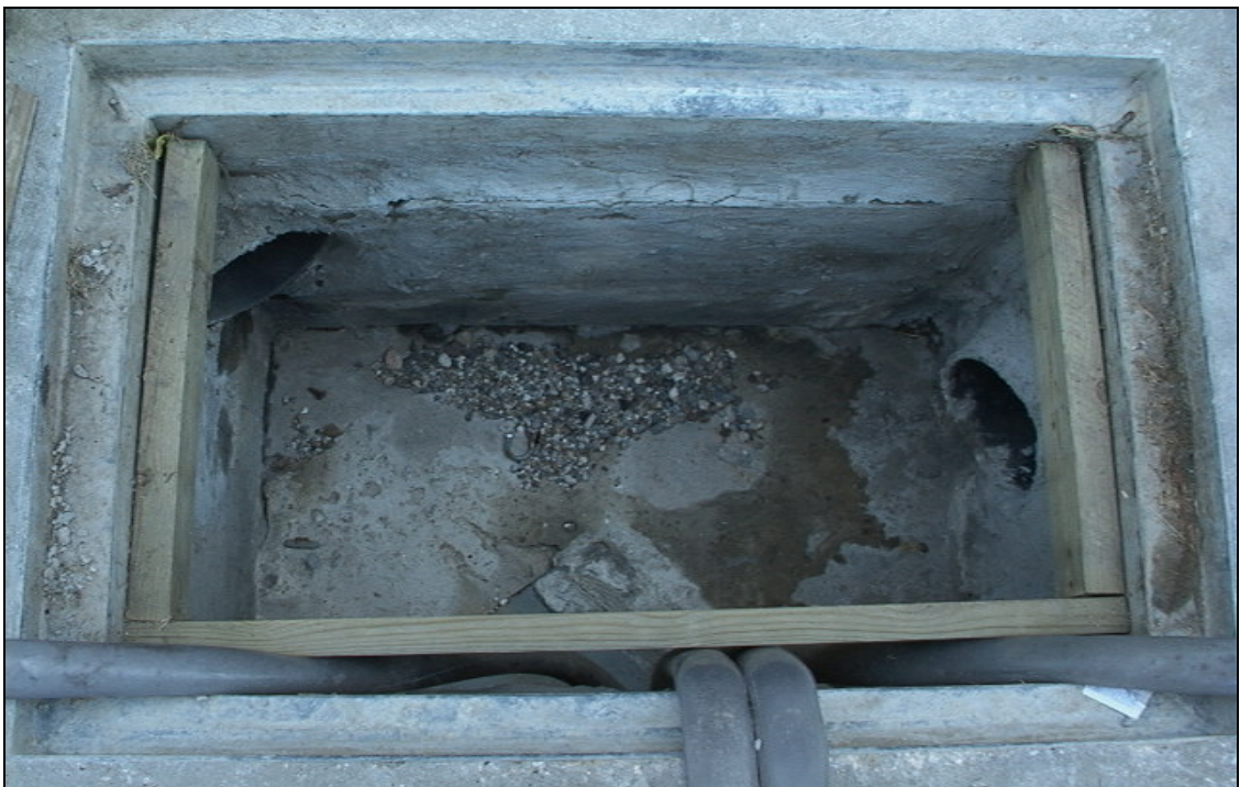
Figure 5: Drainpipes in Manhole from which the Highway Runoff is Collected.
