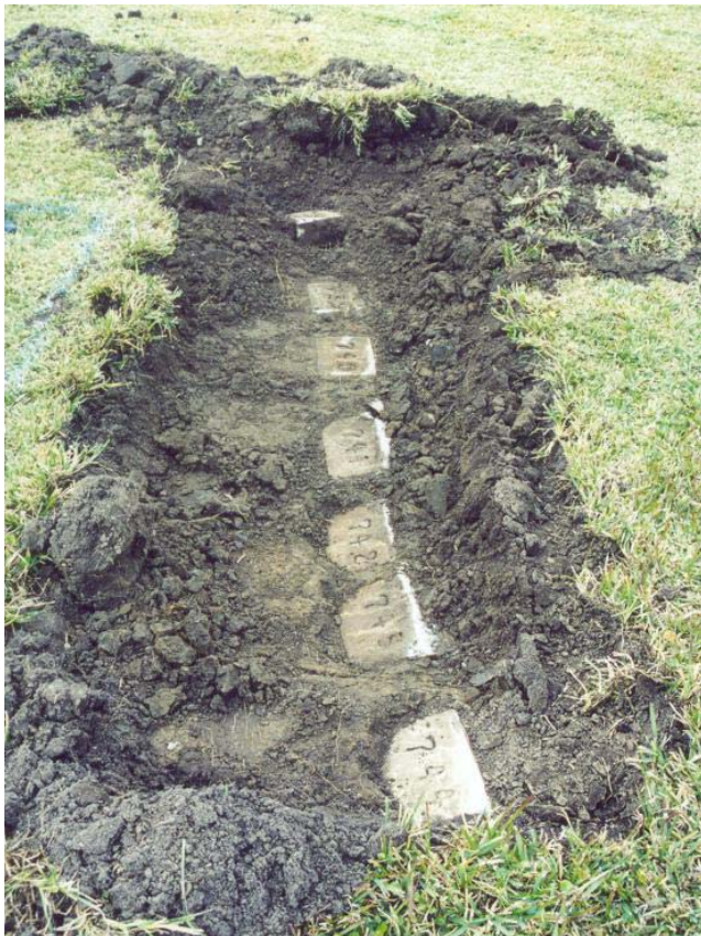
Figures 9a (above) and 9b (left): At depths ranging from 13cm to 19cm rows of cement marker blocks were uncovered.
