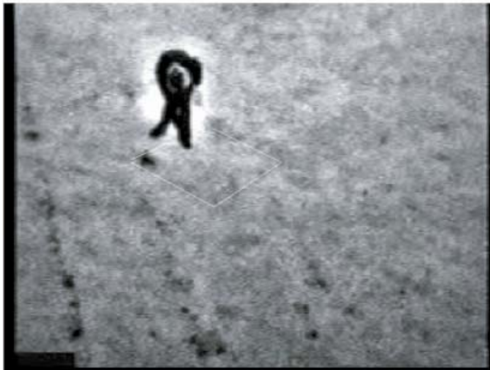
Figure 11. Thermal anomaly (outlined in lower image) in the process of being marked.
