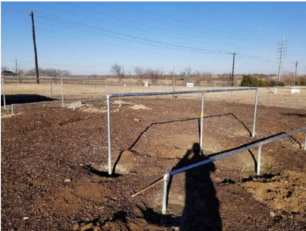
Figure 3.4 : Solar panel mounts
