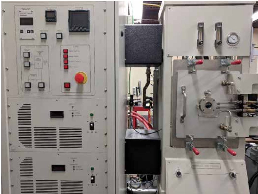
Figure 2 – SPS Furnace and Control Cabinet
