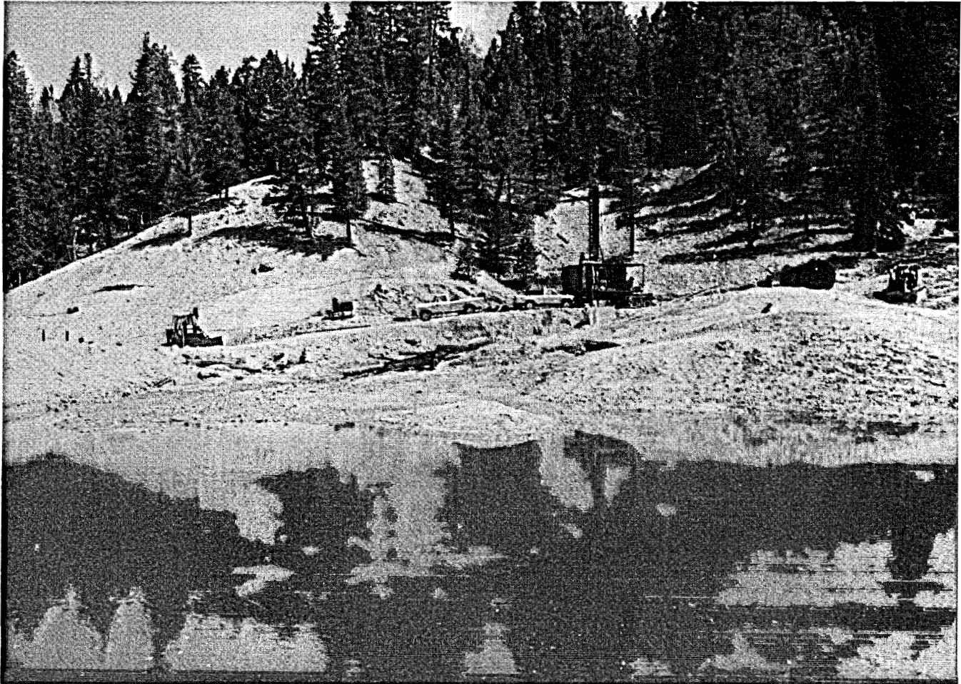
Fig. A-5. Looking east at the diamond core rig during setup over VC-2a, September 3, 1986; storage pond in foreground has pH = 3.
