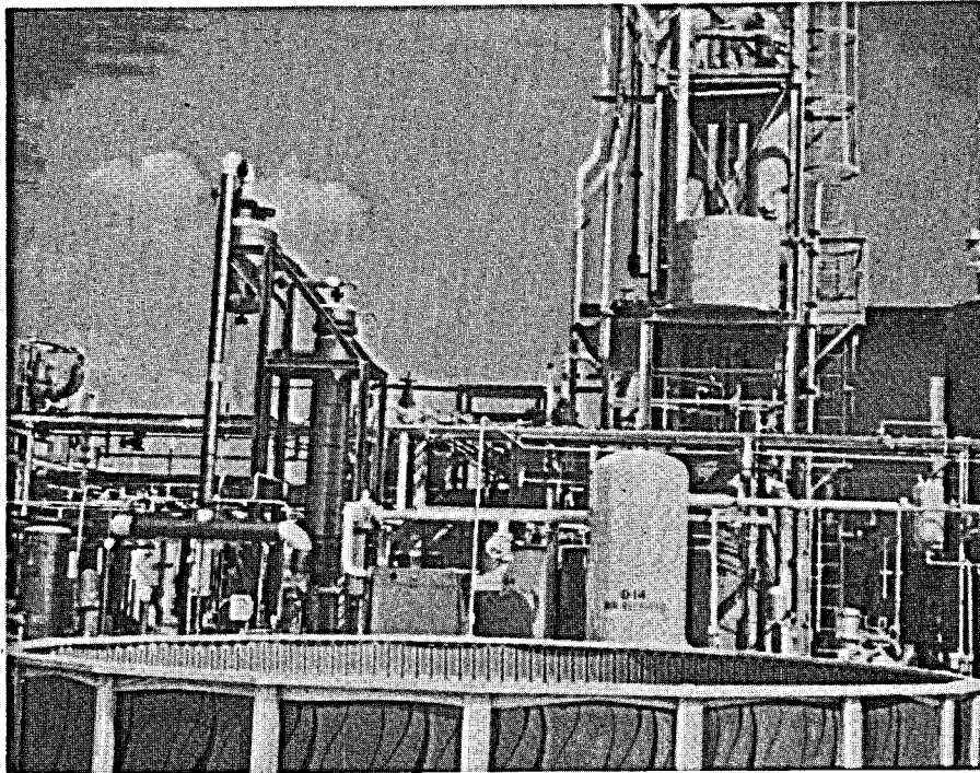
Fig. 18. Dow Freeport facility.
