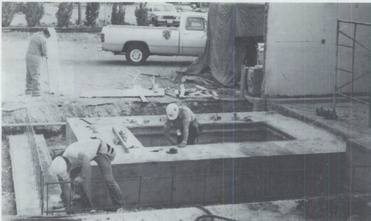
FIGURE 7. The Construction of the Footing for the Shielded Room Moved from the University of Utah
