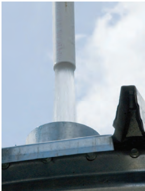
Figure 9.13 Air gap between potable or recycled makeup water and reclaim storage tank
