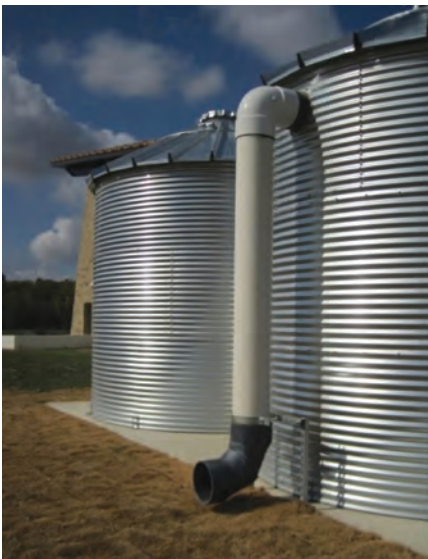
Figure 9.12 Tank overflow pipe
