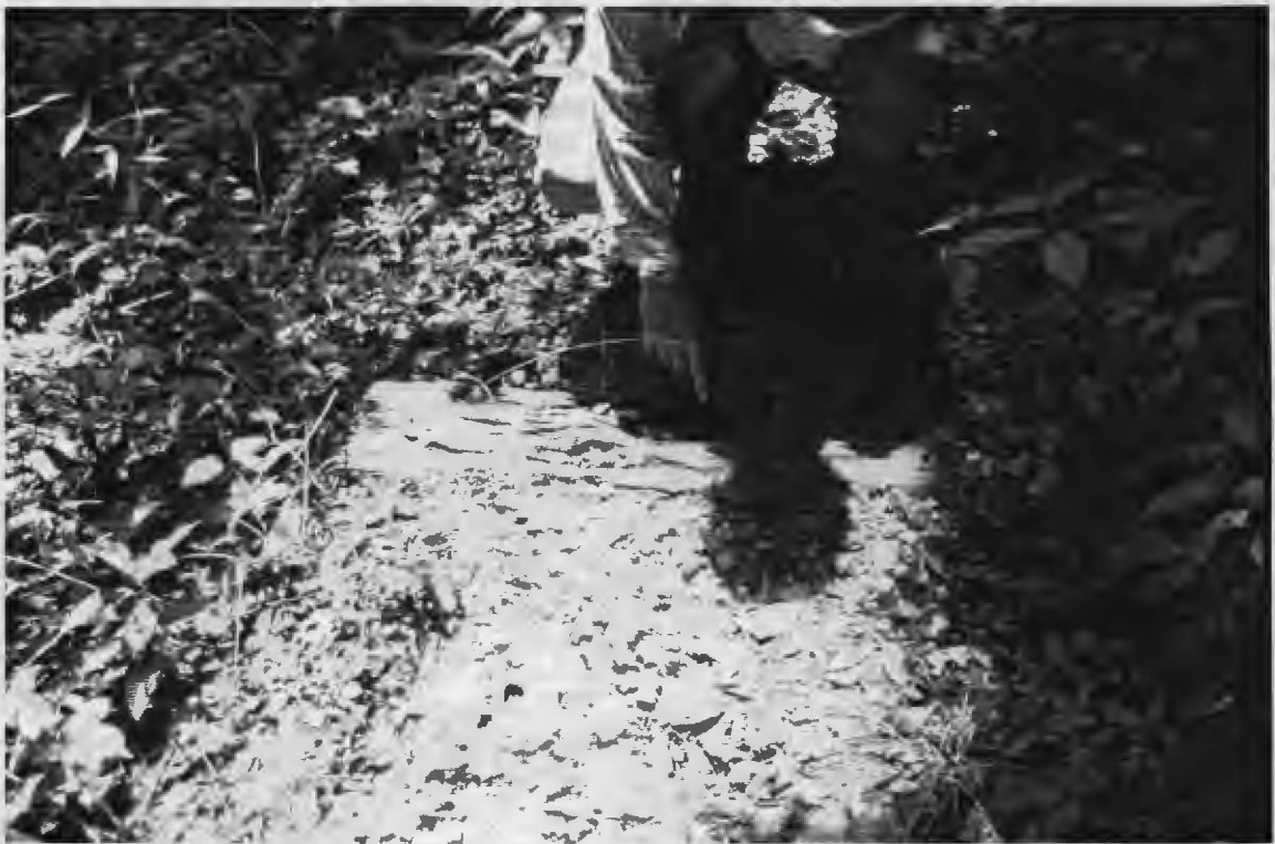
Figure 9.5. Roughly hewn railroad ties laid in gravel on top of a wider (4 m) road bed.
