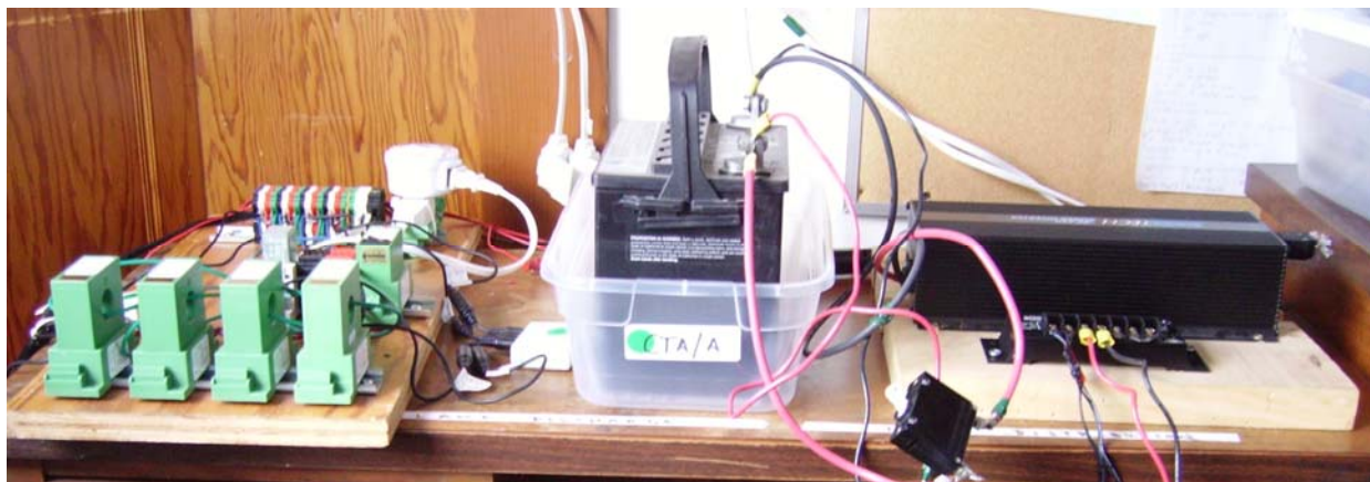
Figure 7. AC Power Supply for Grid Charging. 230V/50Hz pure sine wave inverter (far right), 6 V battery to power the inverter (middle), datalogging equipment (far left).
