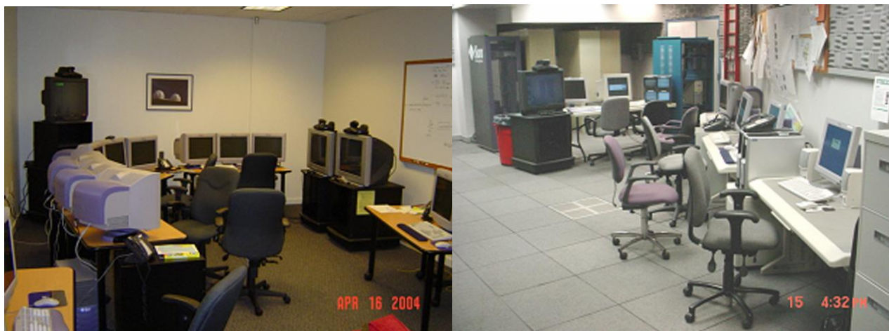
Fig. 9. Headquarters (left) and summit (right) interferometer control rooms.
