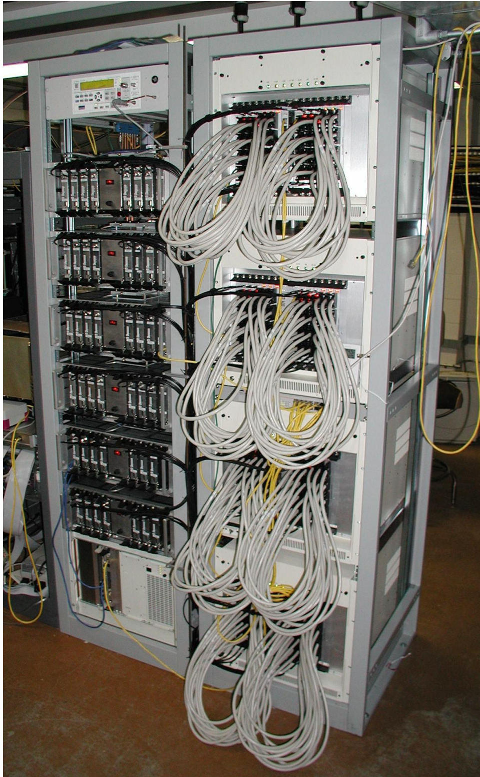
Figure 6. The 4GHz bandwidth COBRA Wideband Correlator System. The analog downconverter system is shown on the left-hand-side of the photo, while the digital correlator is shown on the right-hand-side. The black cabling is for the RF signals, while the lighter cabling is the digital LVDS cabling.
