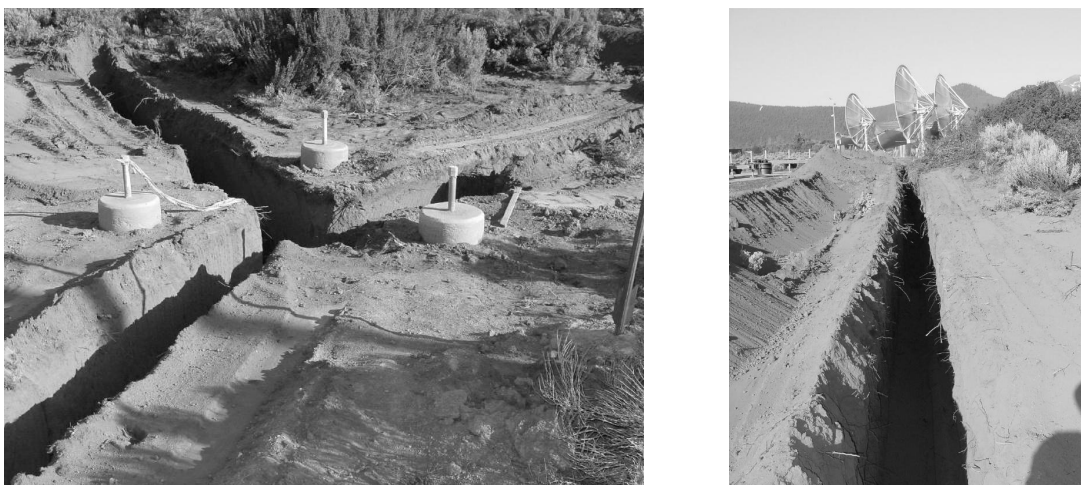
Figure 7: Picture of the trenching threading an antenna foundation (left) and the trench headed towards the three existing ATA dishes. (Credit David DeBoer)
