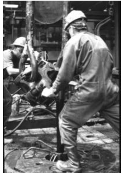
Figure 1.3. Drilling rig floor
