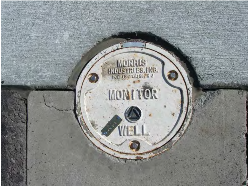
Example flush-mount completion monitoring well with brass ID tag. Many of the monitoring/injection wells at Sites N2, N3, and N7 are installed flush mount in aircraft ramps and taxiways.
