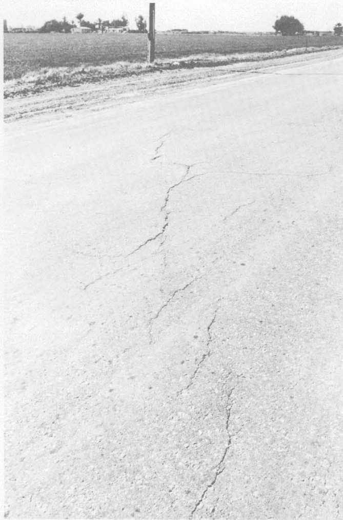
FIGURE 57.— En echelon cracks on Meloland Road first observed following the Imperial earthquake of 1966 (Brune and Allen, 1967a) but slightly widened during the Borrego Mountain earthquake. Fault displacement of about one-half m occurred at this same locality in 1940. Photograph taken April 28, 1968.
