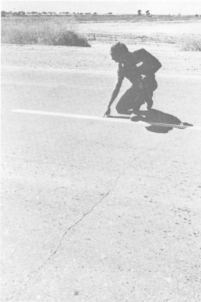
FIGURE 58. — Fresh cracks across Heber Road. Displacement of about 1\frac{1}{2} m took place here in 1940, but no further displacements are known to have occurred here until 1968. Photograph taken April 28, 1968.
