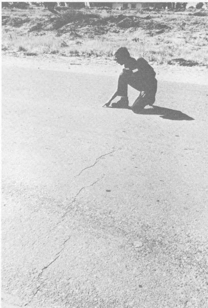
FIGURE 56.— Fresh en echelon cracks crossing Ross Road. View southeast. Photograph taken April 28, 1968.
