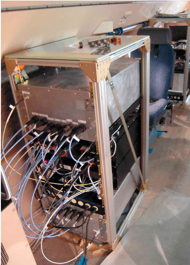
Figure 1. ADELE installed in the GV. The aluminum boxes at top and bottom are the sensor heads; the two computers are the black boxes in the middle of the rack.
