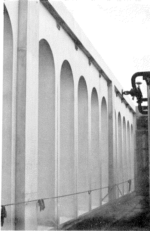
Fig. AV-10. NORTH SIDE ROOF PANEL, LOOKING FROM THE INSIDE OF THE BUILDING. NOTE THE STEEL CONNECTION BETWEEN THE TOP BEAM AND THE PRECAST WINDOW WALL PANELS.
