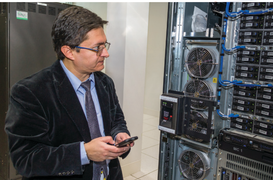
Associate Professor Carlos Caicedo examines hardware in the University's Green Data Center. Caicedo is the curriculum lead for the iSchool's new master's degree in Enterprise Data Systems.
