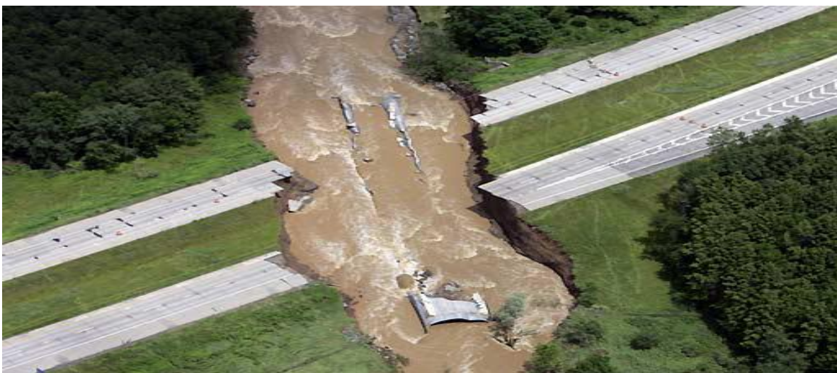
Figure 25: I88 at Collapsed Carrs Creek Crossing on June 28th, 2006 (Geotechnical Engineering Bureau, 2008)
