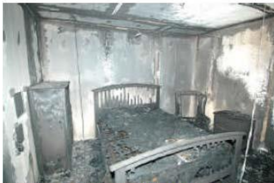
Figure 8. View to SW in cell 3 showing damage to the bed's east side near the door
