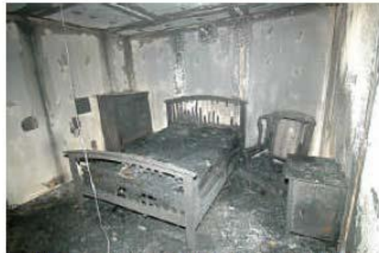
Figure 9. View to SE in cell 3. Note the absence of clean-burn near the origin
