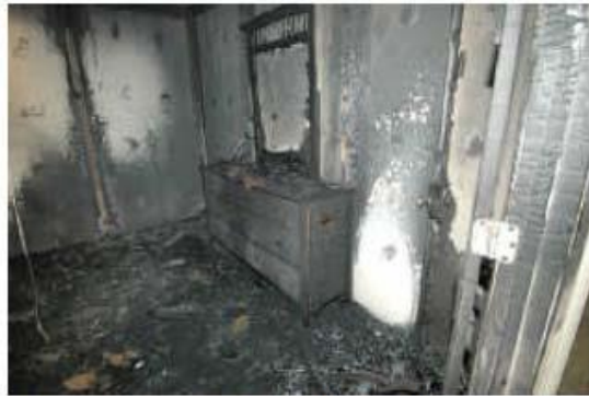
Figure 7. View of N wall of cell 3 through the doorway. Note the area of clean-burn.
