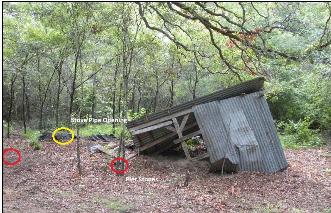
Figure 5.5: Overview close-up of the collapsed structure at the Davis Site (41AN188), facing east. The visible pier stones are in circled red and the stove pipe exit is circled in yellow (S. Loftus).
