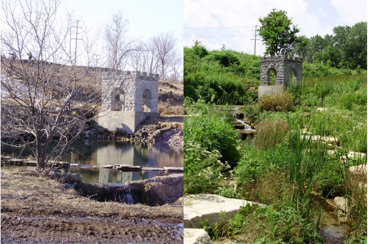
Figure 3.5 The Coldwater Spring springhouse. The photo on the left was taken 18 February 2012 during demolition, and the water in the foreground flowed underground through a culvert. The photo on the right was taken 13 July 2014 after the creek was “daylighted.”
