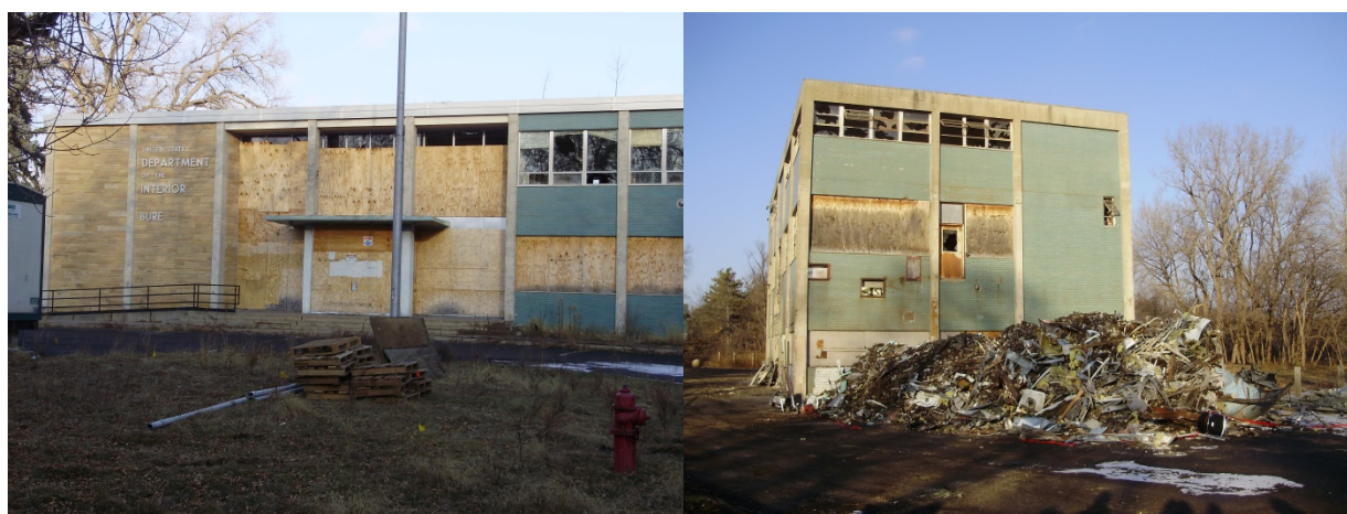
Figure 3.1 Dilapidated U.S. Bureau of Mines buildings. Photos taken 17 December 2011.
