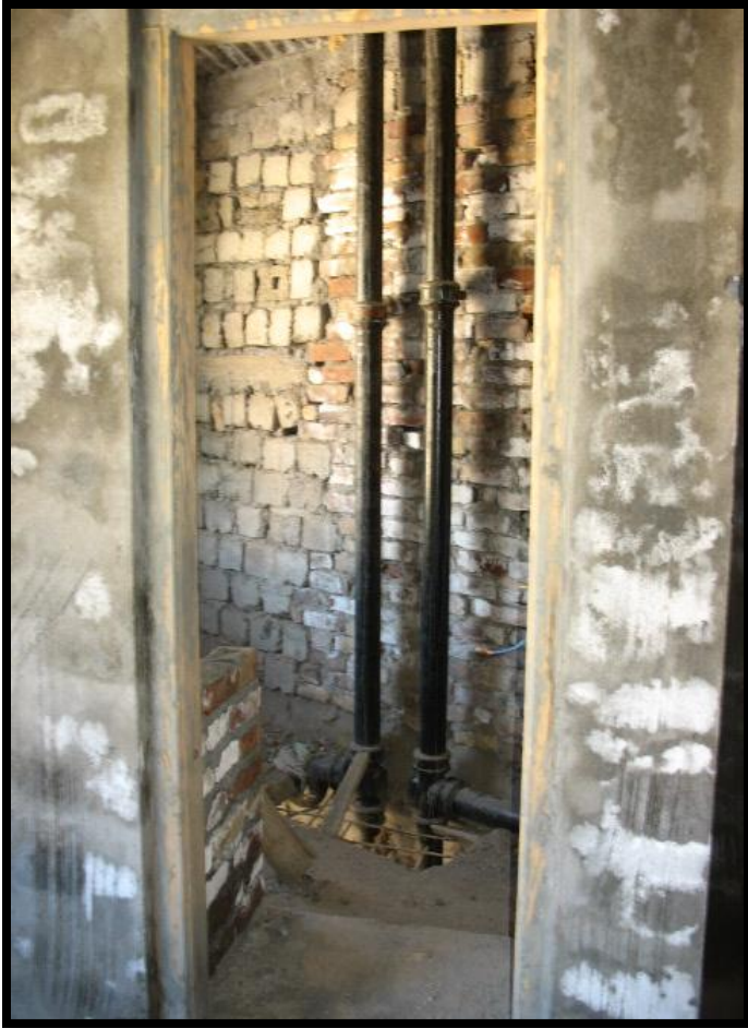
34. Dragon Hotel bathroom before plastering: mud brick, brick, and stone filled in with concrete. Photo by author.
