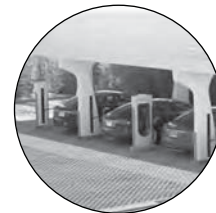
Tesla Supercharger Station Photo Credit : Tesla Motors
