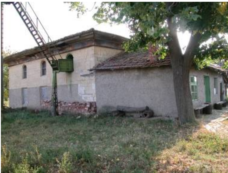
Oblique view from left. Note bricked-in portico, improvised access to minaret, cracks and buckling at left front corner, and laying of brick in an attempt to shore up wall.
