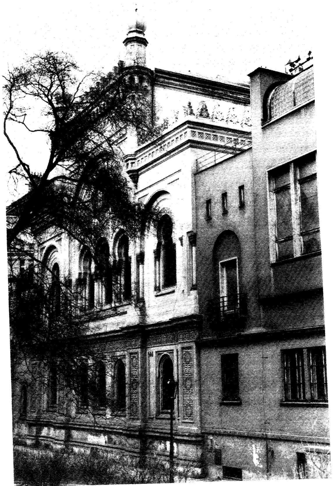
Prague. The facade of the Spanish Synagogue (1867-68) and its adjacent annex, built in the 1930s. Despite some repairs, both buildings are in serious need of restoration. (photo: Rob Cutner)
