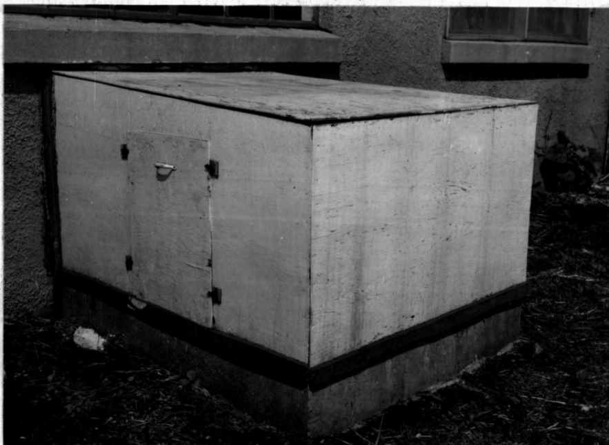
Figure 1. Exterior View of Compressor Housing
