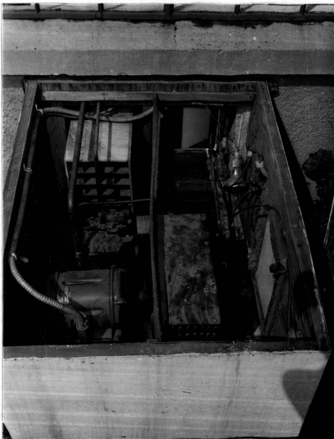
Figure 4. Compressor Housing With Top Removed Showing the Components of the Installation
