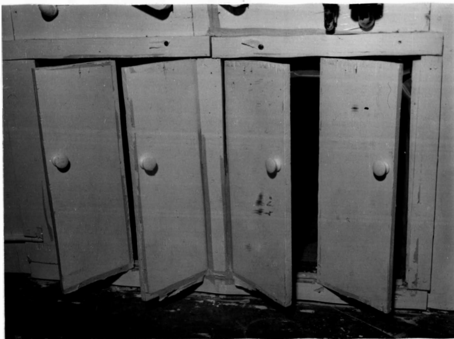
Figure 3. Adjustable Vents Joining the Compressor Housing and Milkroom Viewed from the Milkroom Side
