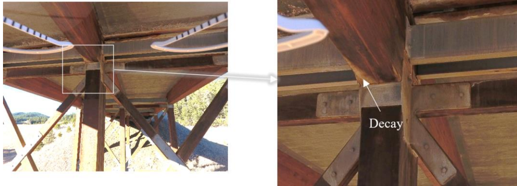
Fig. 4-6. Damage identified on Stringer 2 at Joint 4 captured using UAV (taken by Luis Duque using UAV).
