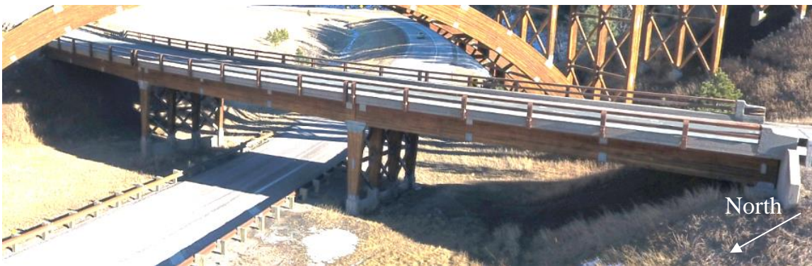
Fig. 2-2. Glulam timber girder bridge overview taken by the drone (taken by Luis Duque).
