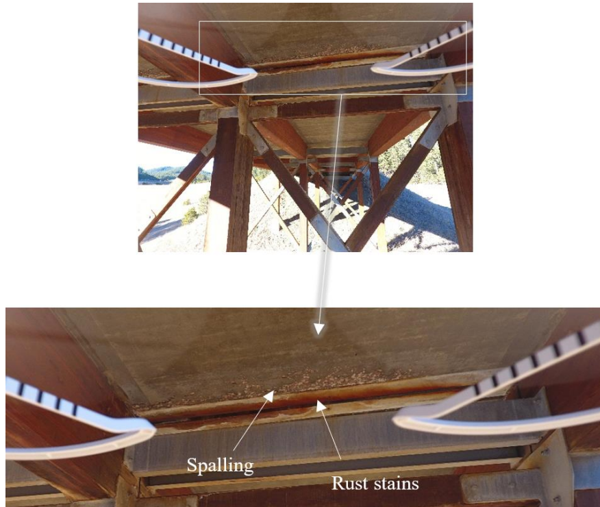
Fig. 4-5. Sample damage on Joint 4 captured with UAV (taken by Junwon Seo using UAV).
