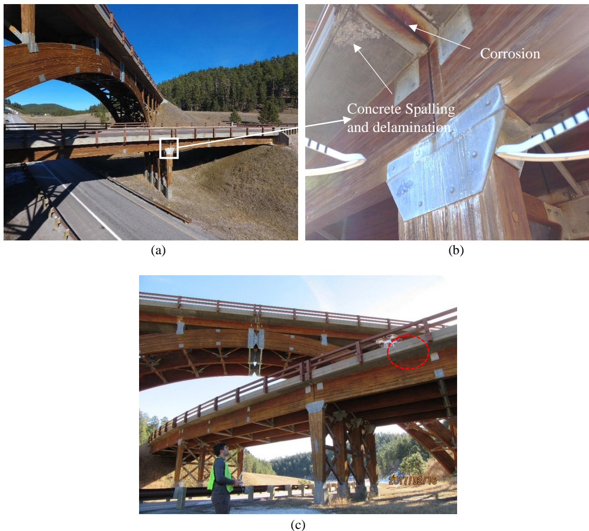
Fig. 2-7. Sample images obtained from the timber girder bridge inspection: (a) glulam girder bridge overview (taken by Junwon Seo using drone); (b) damage on timber girder bridge (taken by Luis Duque using drone); and (c) drone flying near girder (taken by Junwon Seo using digital camera).
