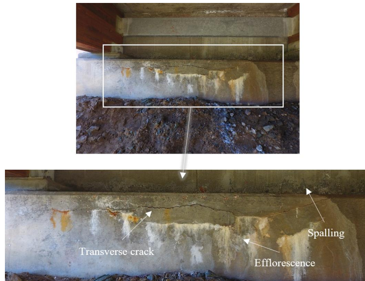
Fig. 4-7. Sample abutment damage detected using UAV on Bay 1 at North Abutment (taken by Luis Duque using UAV).
