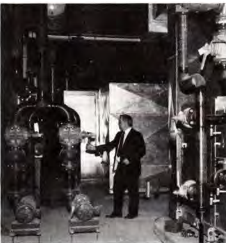
Schmidt turns a valve on a pipe leading from a heating circulation pump. At right is the heating, ventilation, and air conditioning unit for the building.
