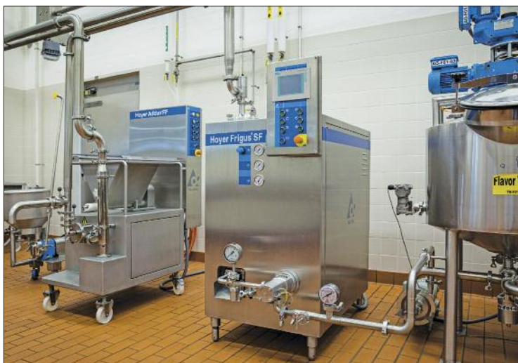
Ice cream making equipment at the Davis Dairy Plant.
