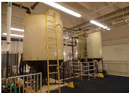
MIEX ® Storage Tanks
