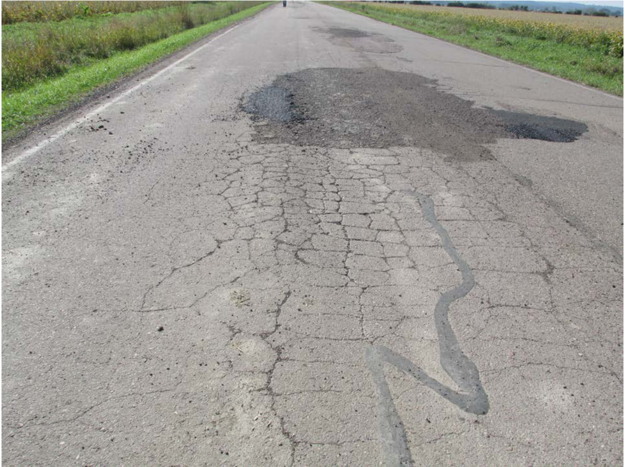
Figure 5.1: Category 1 Pavement Condition – Clay County Saginaw Avenue
