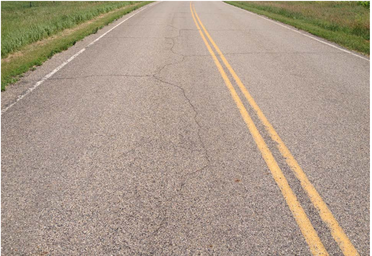
Figure 5.2: Category 2 Pavement Condition - Deuel County Highway 311-Original
