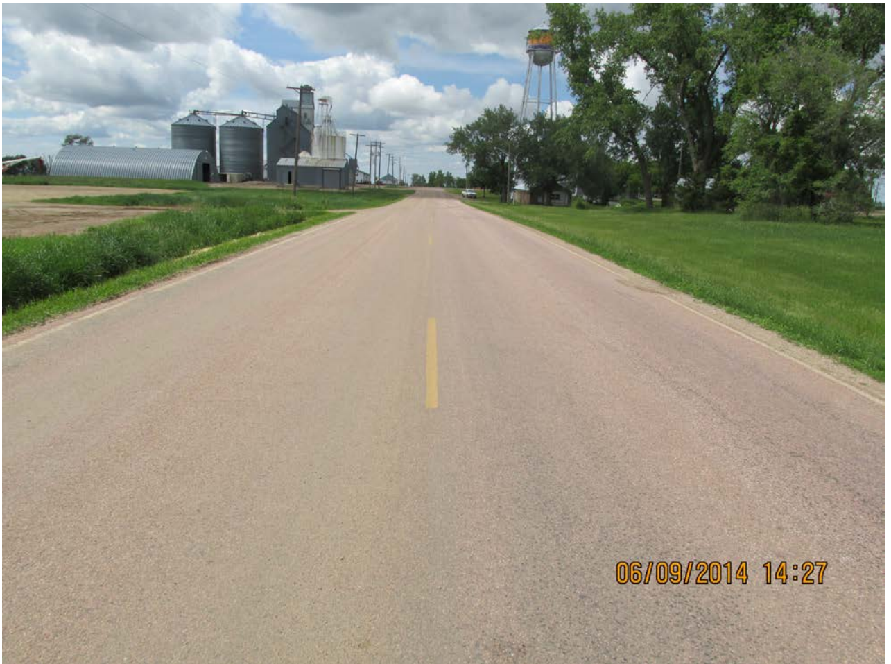
Figure 5.3: Category 3 Pavement Condition–Miner County Railroad St. (Canova)
