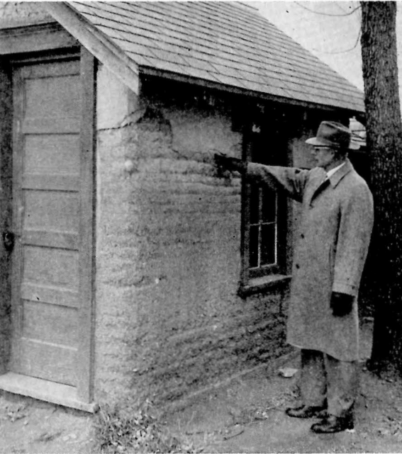
Figure 8. Test wall surfaces that have been painted (gable end) and covered with dagga plaster plus paint (side wall) have failed.
