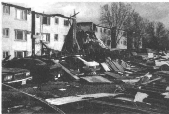
This is the kind of damage seen by SDSU students Drew Schellpeper and Laird Raschke after the May 7 storm
