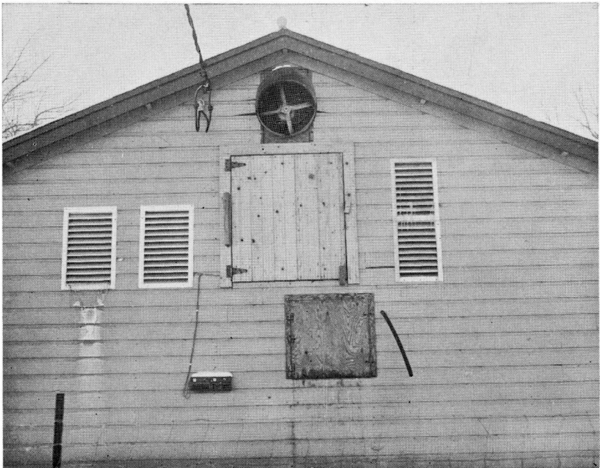
Figure 11. Heat pump mounted in end of poultry house.
