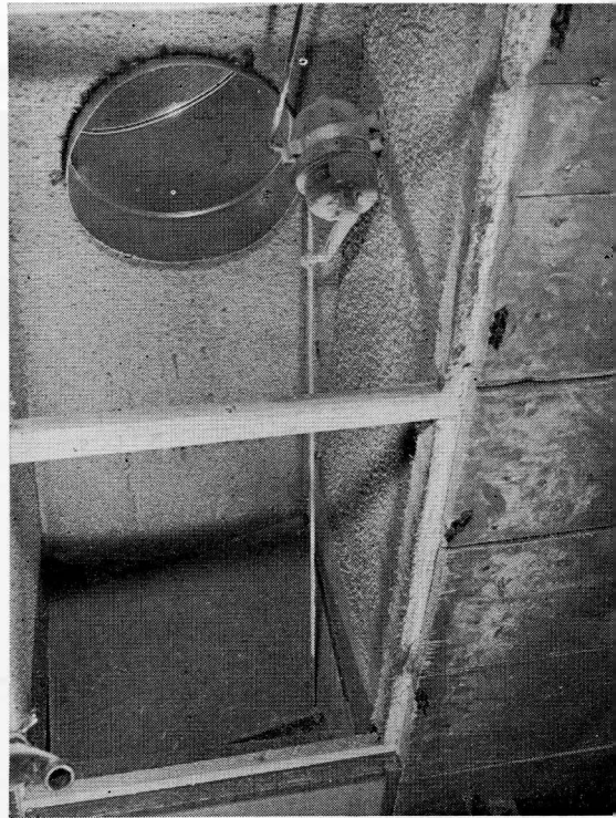
Figure 8. Filter bank with all filters removed.
