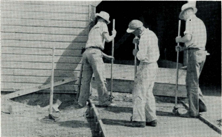
Fig. 17. BUILDING A SOIL-CEMENT FLOOR. The floor is built in strips the same as for concrete. The outside strips are built first. The forms are then removed and the strip between is built. The strips should be the same width so the templates will fit. A width of 5 to 6 feet is best.
