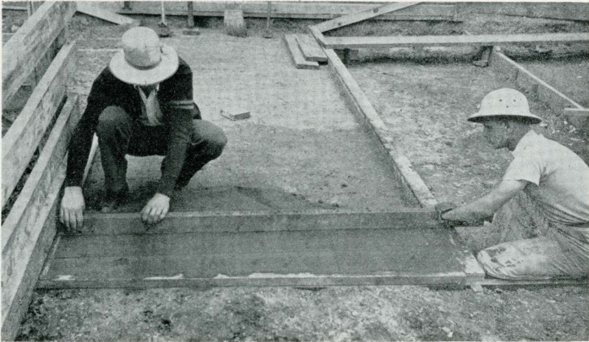
Fig. 18. STRIKING-OFF THE LOOSE SOIL-CEMENT MIXTURE BEFORE RAMMING IT FOR THE TOP COURSE. The back of the template board can be used for this purpose if it has a straight edge. Note the 2x4-inch laid flat for the side-boards. When this is rammed down the floor is finished. See Fig. 17.
