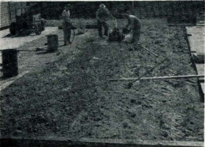
Fig. 9. Mixing in a measured amount of water after the aggregate and cement have been mixed. Speed counts here. The mixed concrete should be leveled within 30 minutes after water is in contact with the cement. A strip of floor of a size that can be leveled within this time limit should be mixed at one time.
