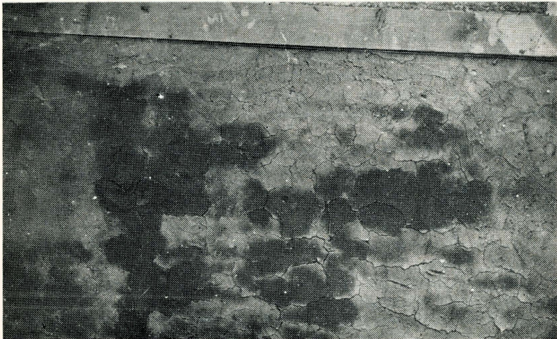
Fig. 7. An Example of Dagga Plaster Containing Too Much Clay and Not Enough Sand.
