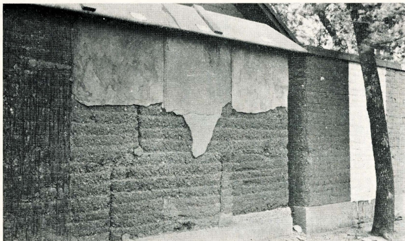
Fig. 21. Plaster Panels Applied Without Any Bond.
