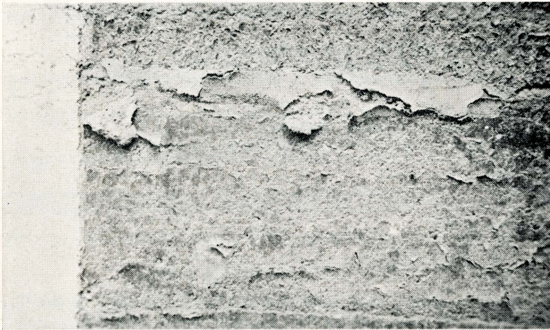
Fig. 19. A Typical Failure of a Transparent Paint.
