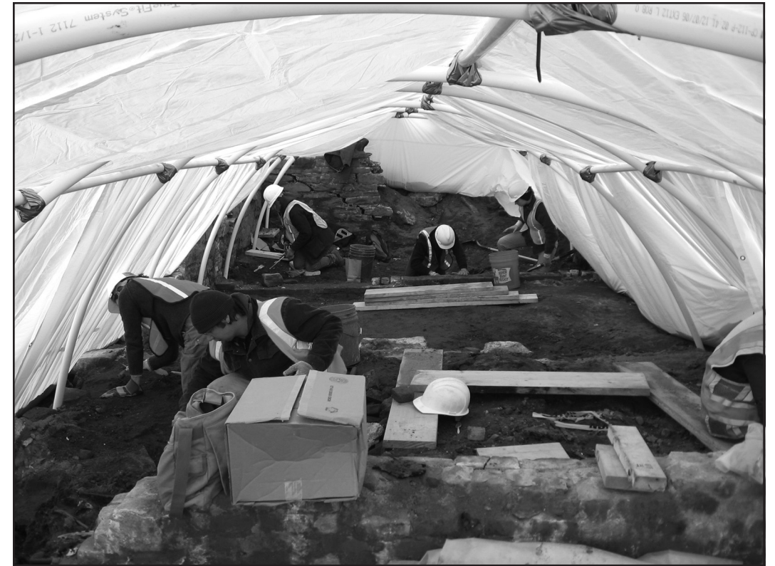
Figure 3. Excavating the burial vaults under the temporary shelter. (Photograph courtesy of URS Corporation.)
