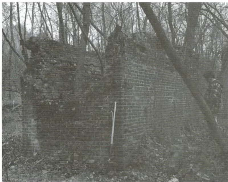
Figure 18. This photograph shows the closed end of Feature A, located within the remains of the Ice House Site B (the P. McCabe & Co. Ice House) powerhouse. The narrow brick structure may have housed the steam engine boiler and firebox. The view is towards the north.
