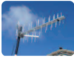
Figure 5: The new Stoke sector antenna
