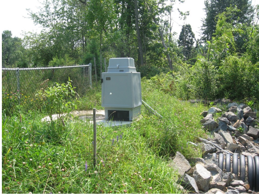
Figure 4: Teledyne ISCO 6712 Refrigerated Sampler installed at effluent location of subsurface gravel wetland.
