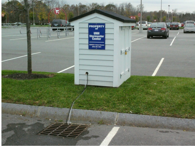
Figure 3: Influent monitoring of direct runoff sampling installation
