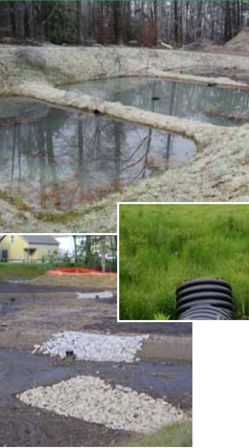
Subsurface Gravel Wetland systems continue to offer superior treatment for common stormwater pollutants and unparalleled treatment of nutrients.
